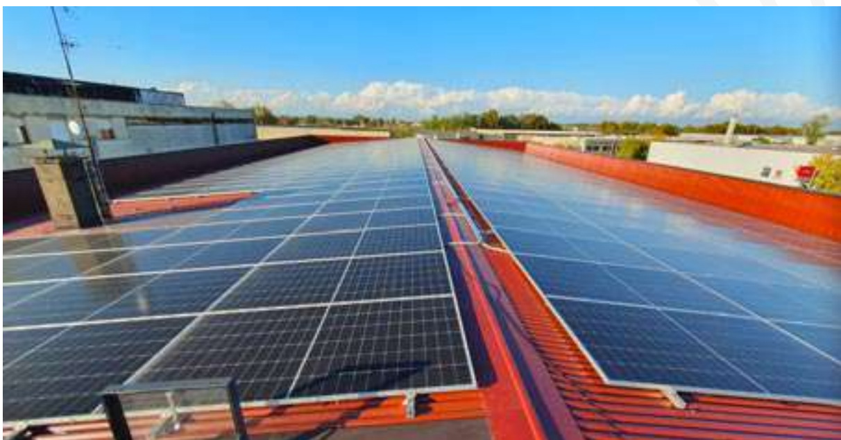
130 kW, Porto Mantovano, Mantua, Italy.
