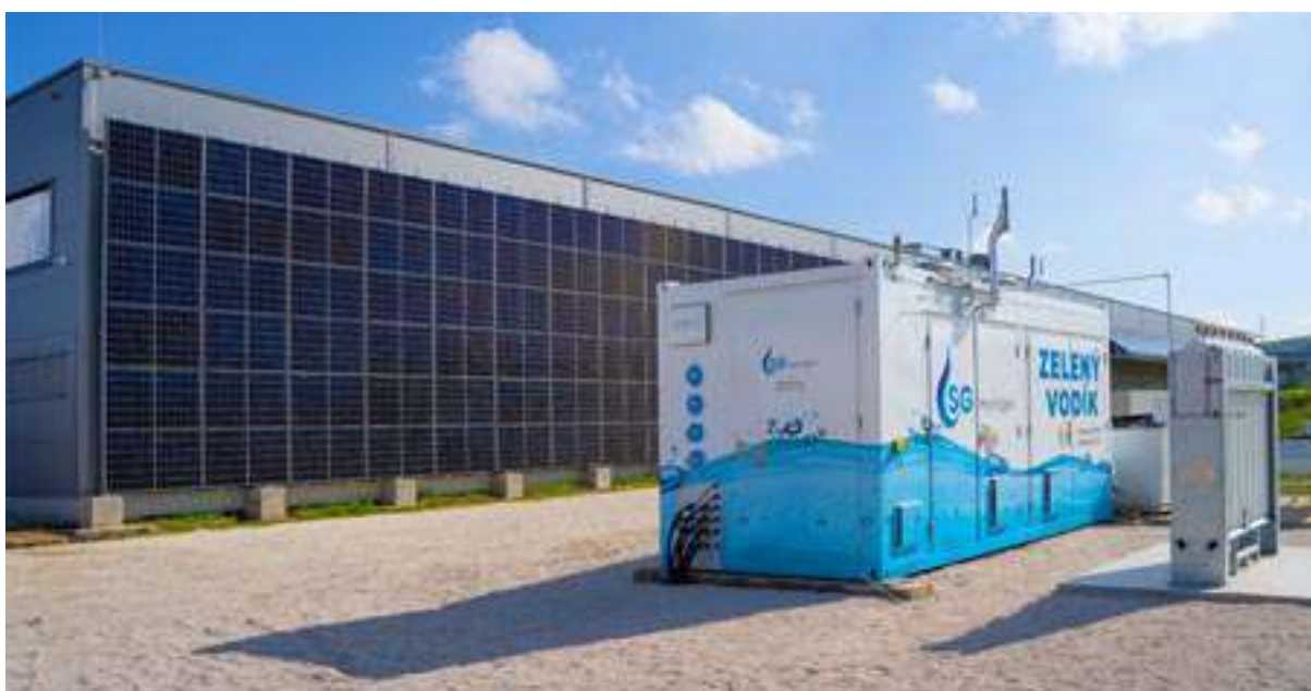
PV + hydrogen project launched in November 2023.
